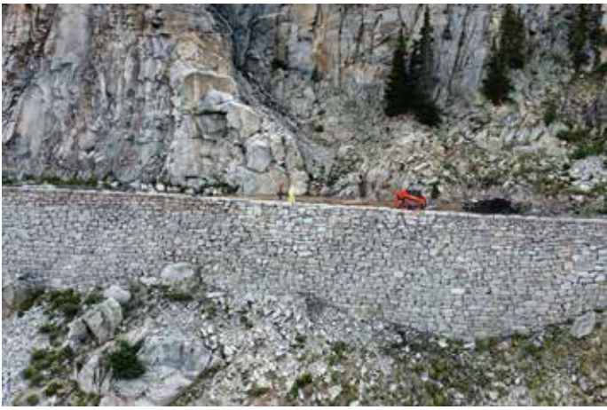
The historic Alpine Tunnel Palisade Wall was reconstructed in 2024. The wall was originally built in the 1880s as part of the Denver, South Park & Pacific Railway and today serves as a popular access for visitors to the Alpine Tunnel Historic Site and recreation opportunities on the Gunnison National Forest.
