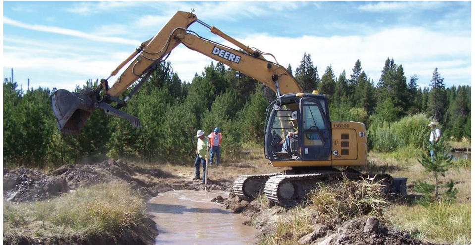
Rebuilding a stream channel to restore connectivity for bull trout, made possible by CFLR. © Craig Bienz
