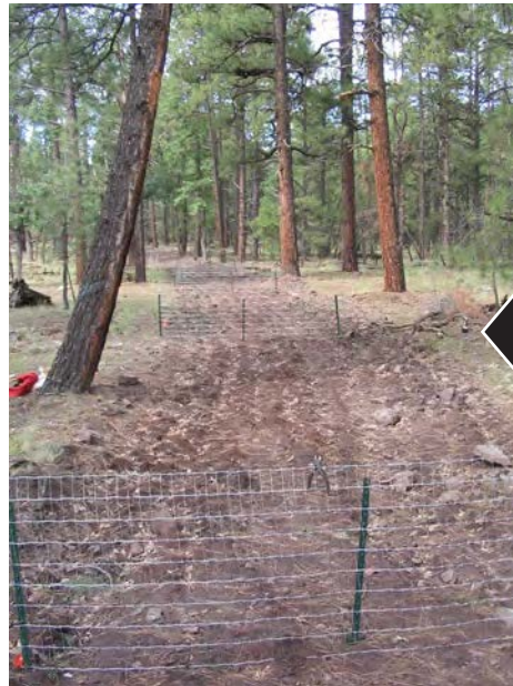
This decommissioned road has been gated to prevent future vehicular travel and facilitate ecosystem restoration. Photo by Joseph Trudeau
